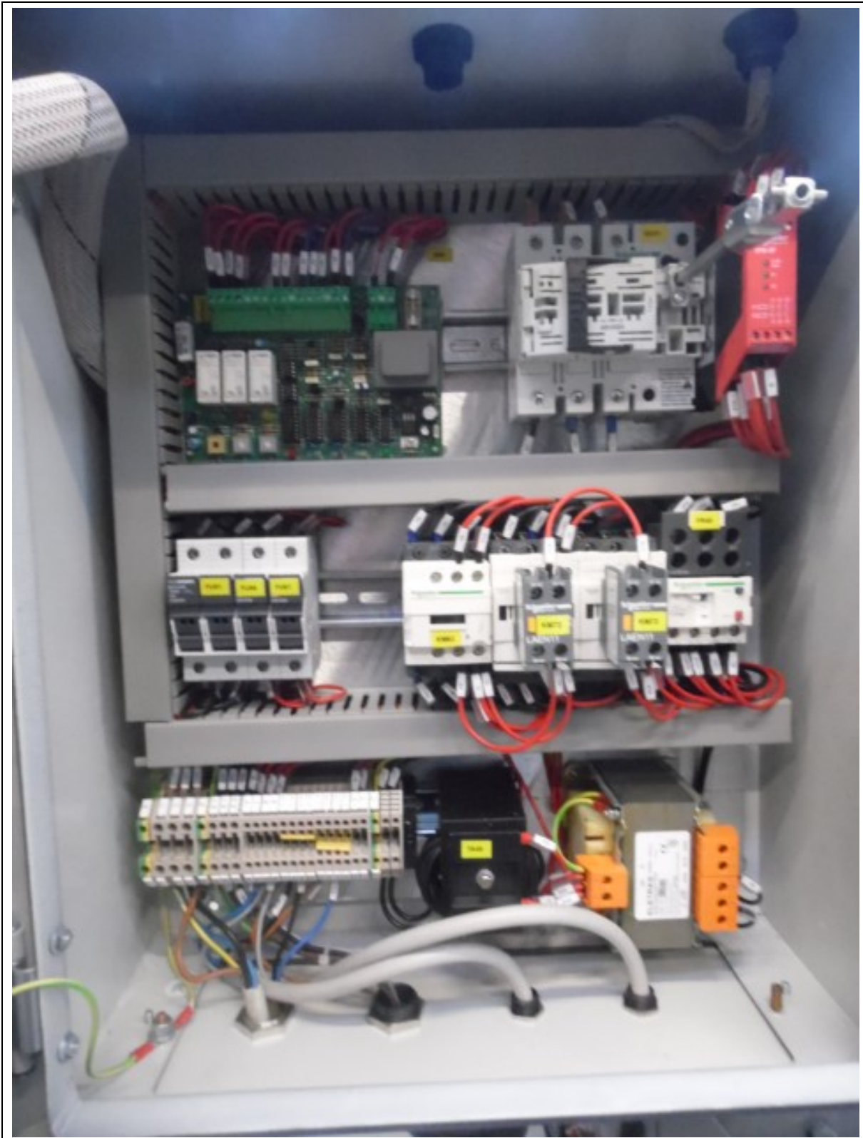
Figure 6-2 – Electric switchboard internal view (Current supply)
